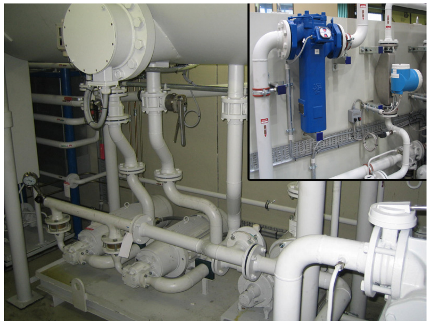
Vacuum oil station, installed underneath vacuum oil tank, and vacuum oil distribution with filtering, flow monitors and pressure control
